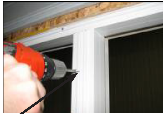
Screw the left and right mull post covers onto the wood mull post. Press the mull post cover tight to the wood mull post when screwing it so the mull cap will properly fit the locking points in the next step.
